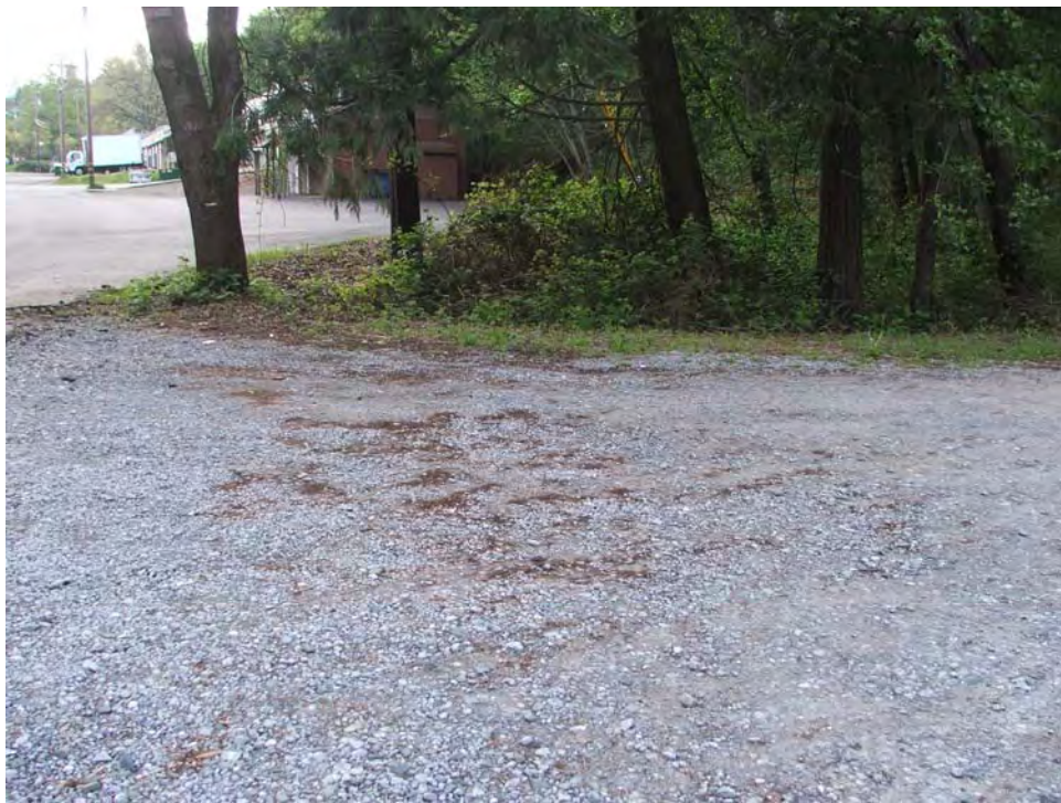
Photograph 9. Culverted area upstream of Canyon View Drive, previously filled crossing in the foreground.
