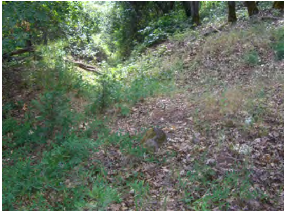
Figure 8. Main ditch blockage.
